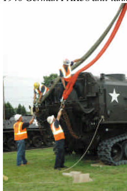
4. From left, riggers Ben Thiesing and Joe Santos, crew chief Vic Abrams and project manager Mike Sturgill attach chains to heavy duty lifting straps before lifting “Tiny Tim” - a Vietnam Era self-propelled Howitzer with a sharp collar weighing more than 90,000 pounds.
